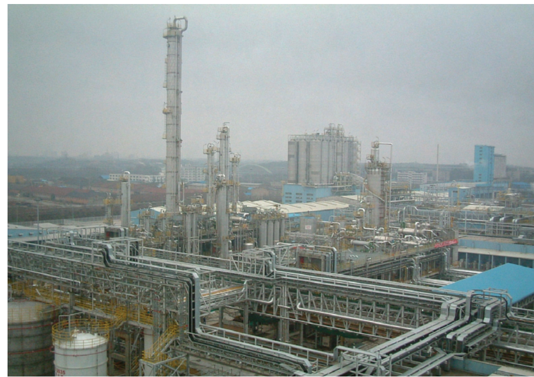
Toyo-China built this OXO alcohol plant in Nanjing for BASF-YPC.
